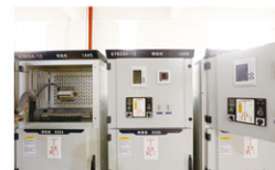
泄压装置 Pressure releasing device
