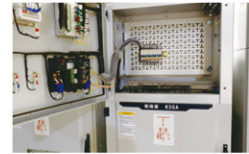
D 继电器仪表室 Relay instrument chamber
